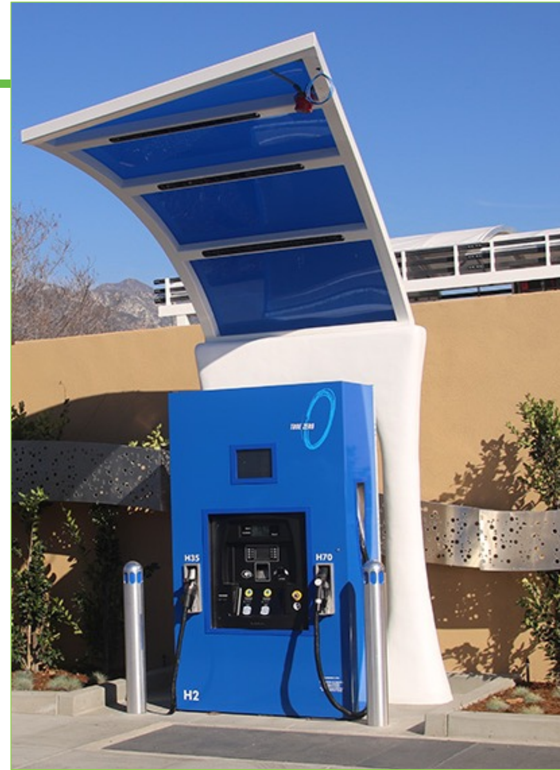
H2 fuel dispenser
